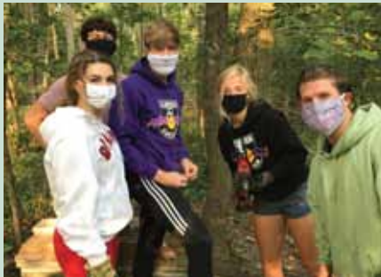
Masked students, tools in hand, build a pedestrian bridge for the trail
