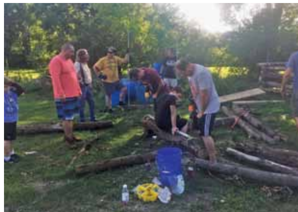
Crib builders hard at work using methods and templates perfected over years
