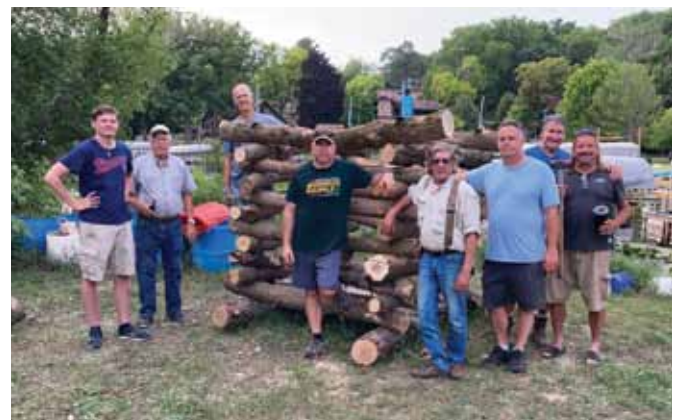
Some of the strapping young men who helped with 2021 crib building. They need your help in 2022 to continue this important program!
