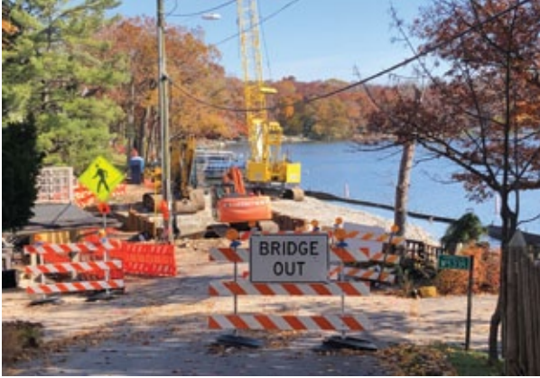
...and so it begins, replacement of the bridge that has served our community since 1915.
