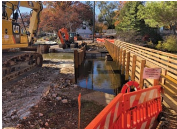
On the right is the pedestrian/golf cart access walkway for Island residents to use during construction.
