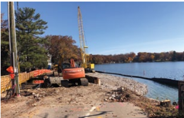
On the right is the temporary gravel roadway for construction equipment to use.
